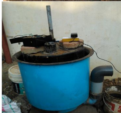
Fig.5 The Installed Biogas Plant
